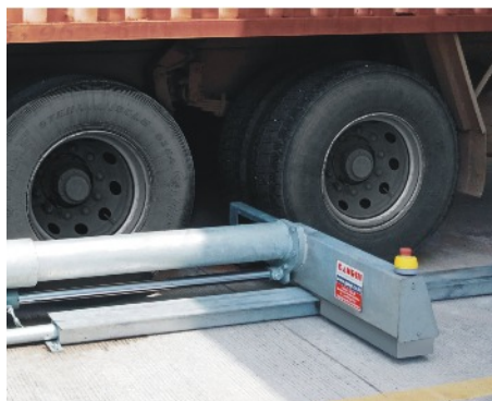
Wheel-Block Vehicle Restraint System
